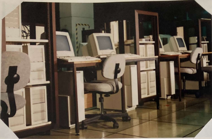
A gaggle of applications servers. Although physically together each is connected to a different building network.
