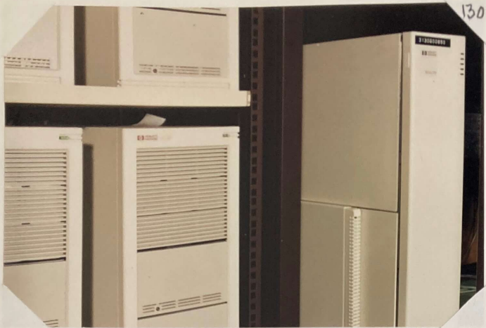
glen Unix applications server for workstation cluster in Herschel Building
